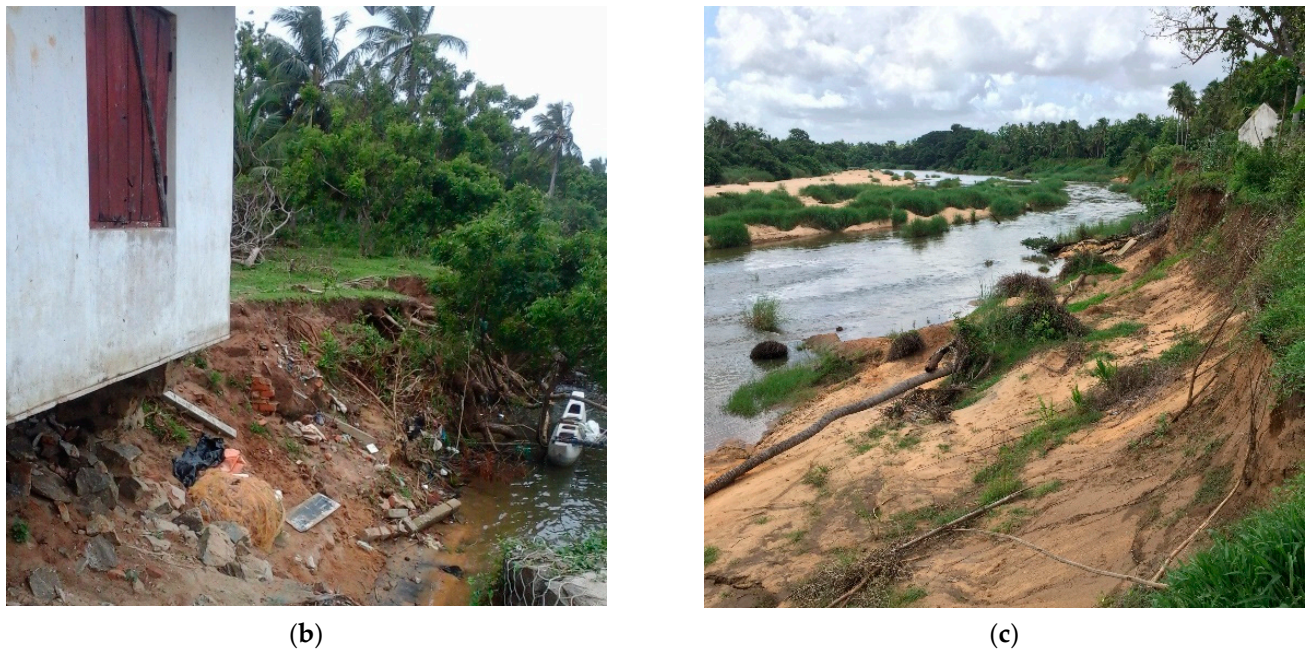
Figure 1. River meandering behavior: (a) meandering behavior and sediment deposition along the Deduru Oya (source: Google maps); (b) eroded riverbanks and damaged houses (photo credit—D.C.H); (c) meandering bend (photo credit—D.C.H).
