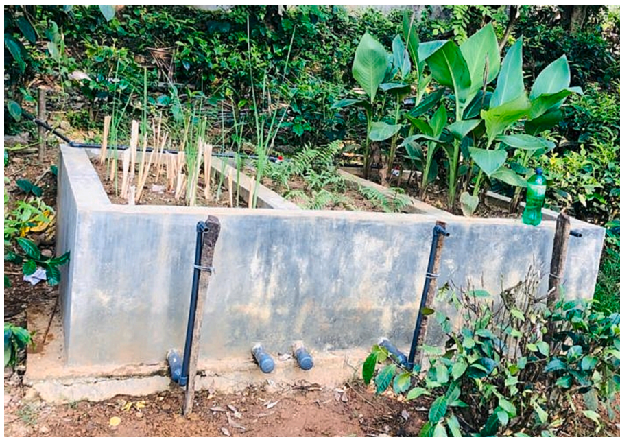
Fig. 4. Final arrangement of VFCW.
