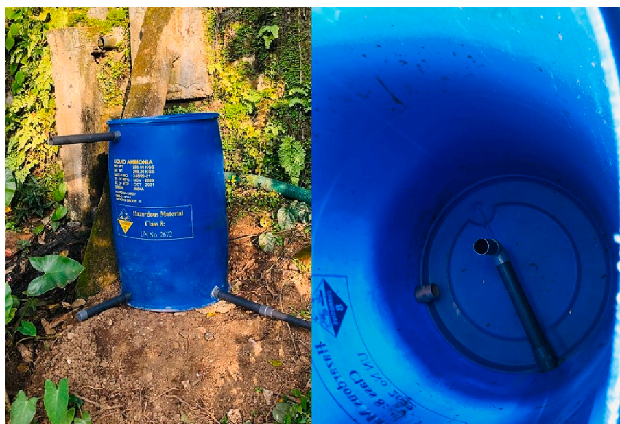
Fig. 3. Retention tank Setup.
