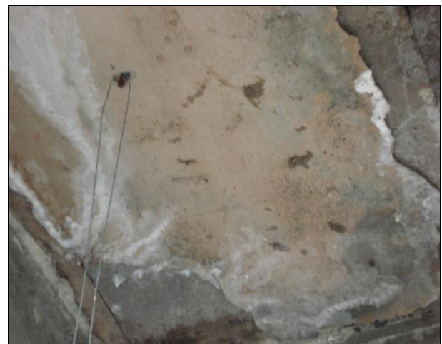
Fig. 5 Efflorescence on slab of Building A.
