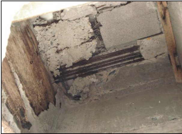
Fig. 6 Corrosion of slab reinforcement of Building A.
