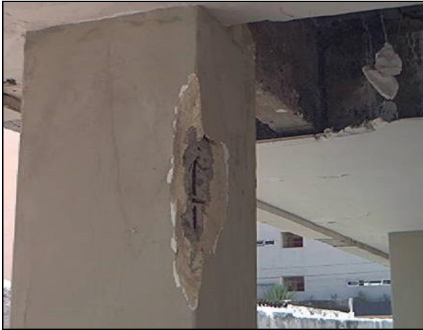
Fig. 8 Detachment column due to reinforcement corrosion.
