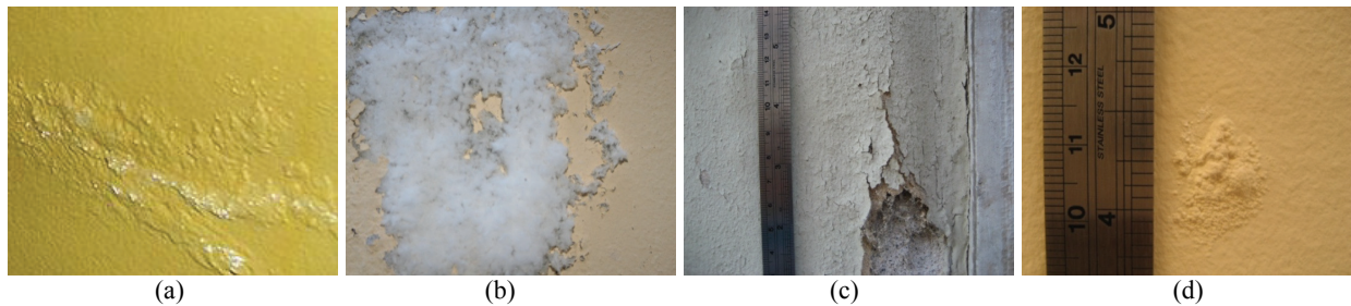
Fig. 8 Common defects in painted interior walls: (a) swelling; (b) efflorescence; (c) cracking; (d) blistering.
